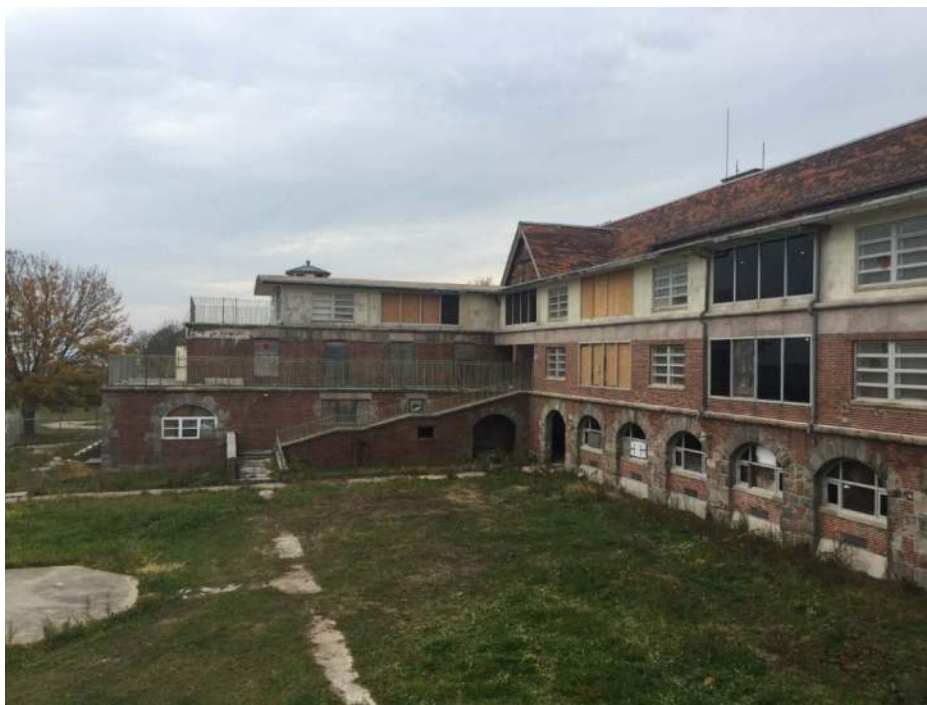
Photo 3-13. Terraces along Main Hospital, allowing multiple patients exposure to the outdoor elements and views of the ocean
