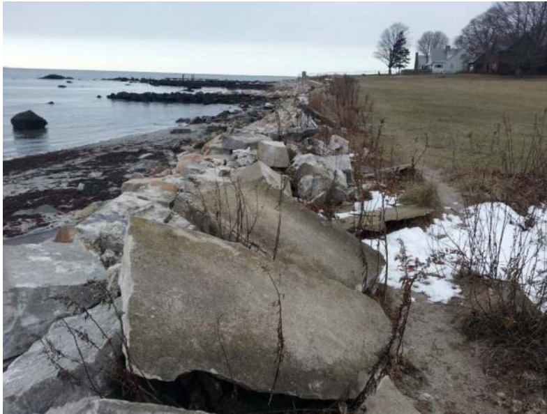
Photo 3-6. Westerly view along broken seawall section
